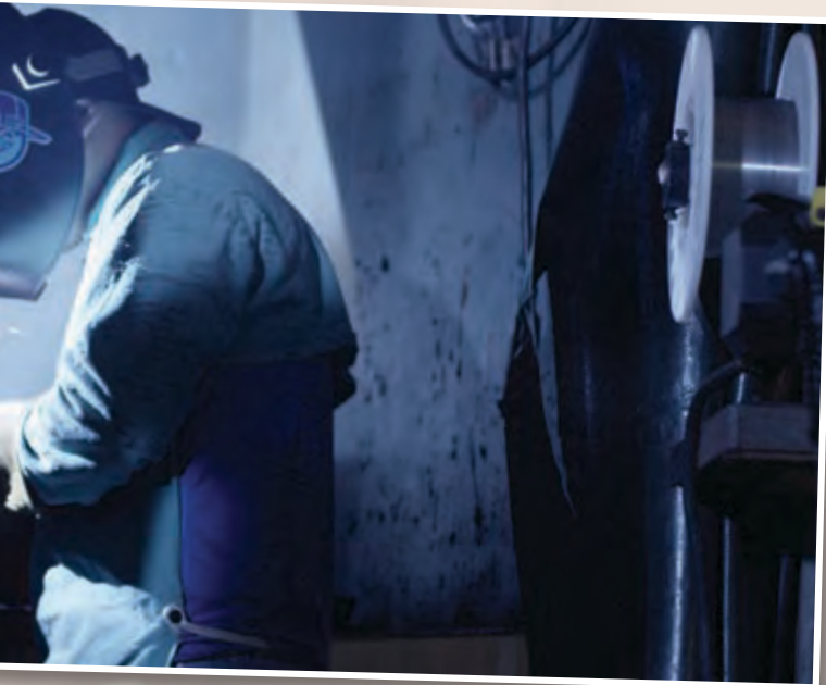
Welding programs are essential to address the workforce needs of the River Parishes region.
